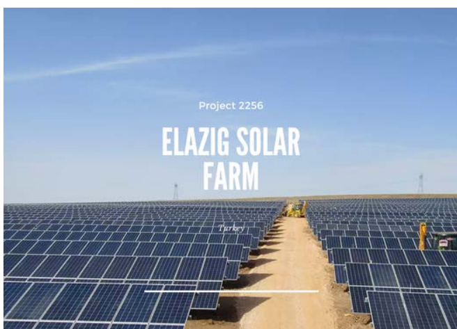
Project 2256: Elazig Solar Farm in Turkey
